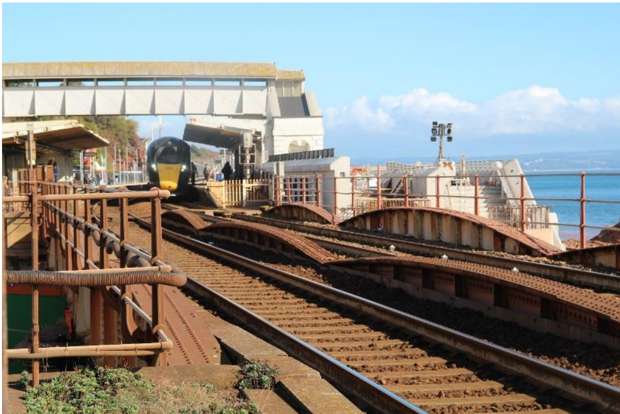
The coastal railway line at Dawlish Station is undergoing major coastal reinforcement works.
